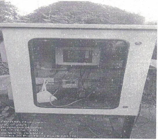
View of Dysfunctional OCEMS of 18 MLD STP, Sector 20, Panchkula (Haryana)
