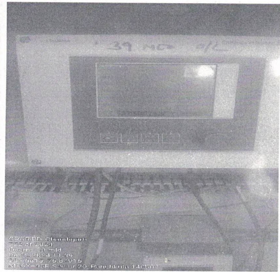
View of OCEMS of 39 MLD STP, Sector 20, Panchkula (Haryana)
